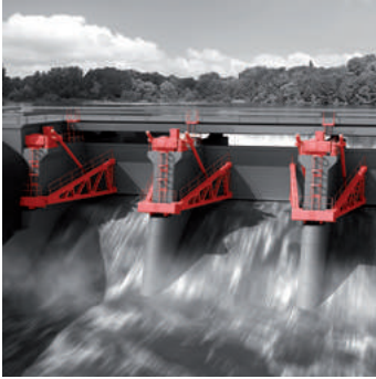
Hydro-electric power stations
